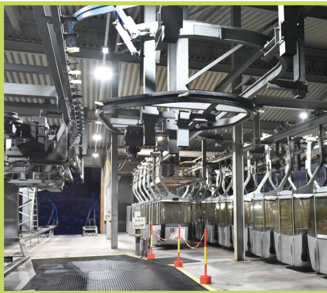
DeltaLUXX - Cable car lighting
