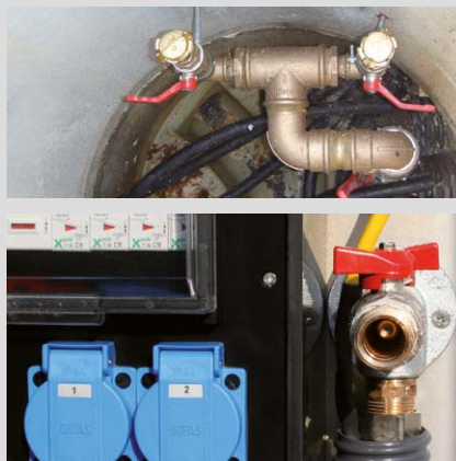
Water supply in / on the shaft or water connection at the shaft cover.
