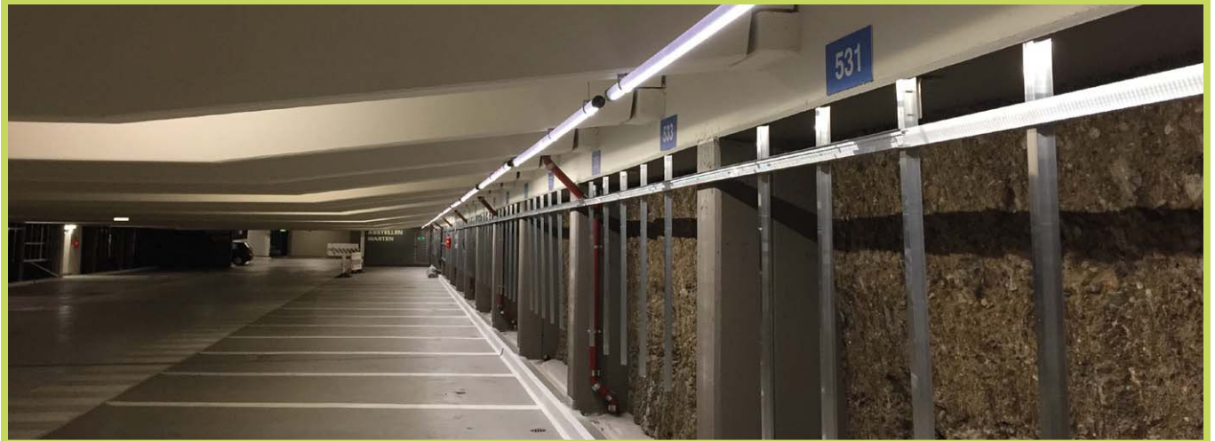
StreamLED Power - Underground garage lighting
