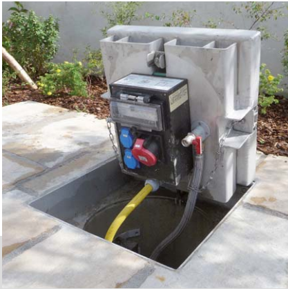
Market town of Schneegattern: Under-ground energy system PIAZZA 540 with two cable outlets and water connections.
