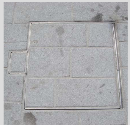
Replenishing the filling tray with filling material adapted to the particular environment (asphalt, concrete, granite, Porphy, and many others ...).
