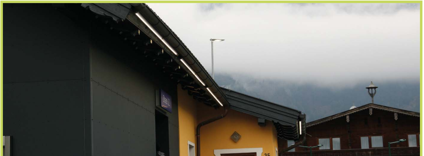
StreamLED Power - Bus stop lighting
