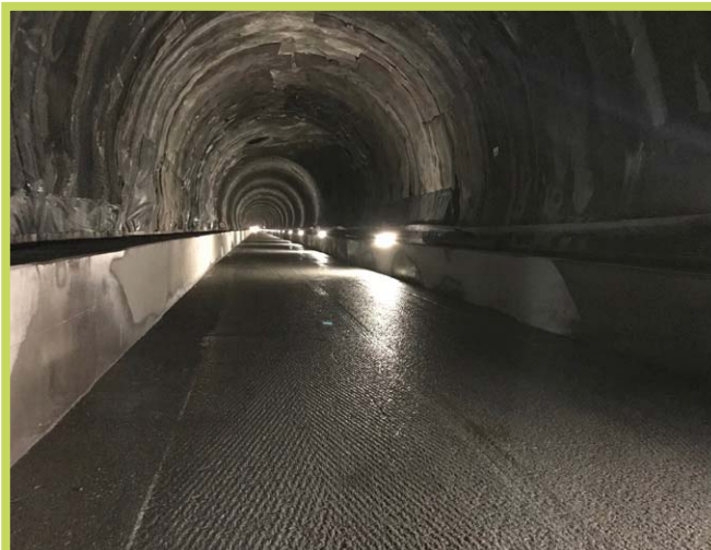
StreamLED Power - Tunnel lighting
