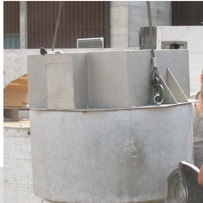
The stainless steel construction, mounted onto the concrete ring, is prepared for installation. Openings for supply cables need to be cut out of the concrete ring.
