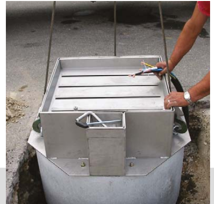
Dropping down of complete unit into the prepared casting pit with suitable lifting aid (crane).
