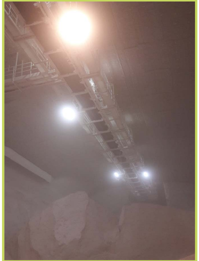
DeltaLUXX 2 HT - Lighting salt works
