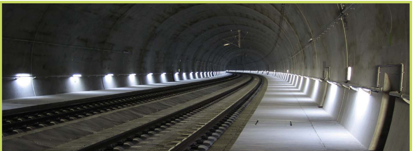
AmbitLED - Lighting the railway tunnel
