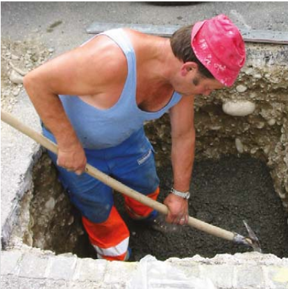
Drawing out of casting pit on the basis of the required dimensions. Installation of a proper foundation as well as a drainage system.
