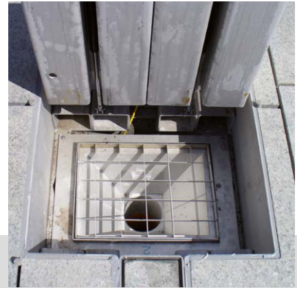
New place in Klagenfurt: Sewage pit with grill. The shaft can be closed while the waste water hose is used.
