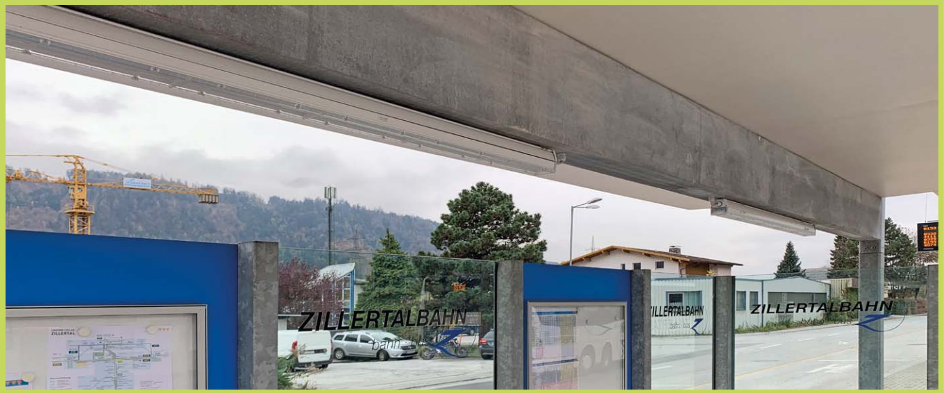
Industry Track LED - Platform / bus stop lighting
