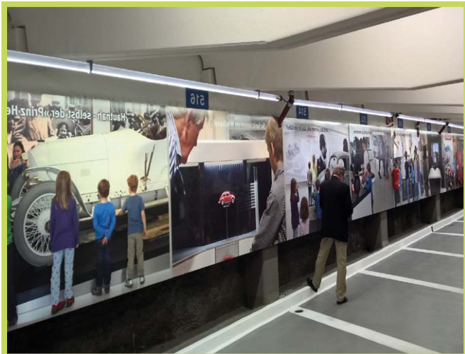
StreamLED Power - Underground parking garage lighting
