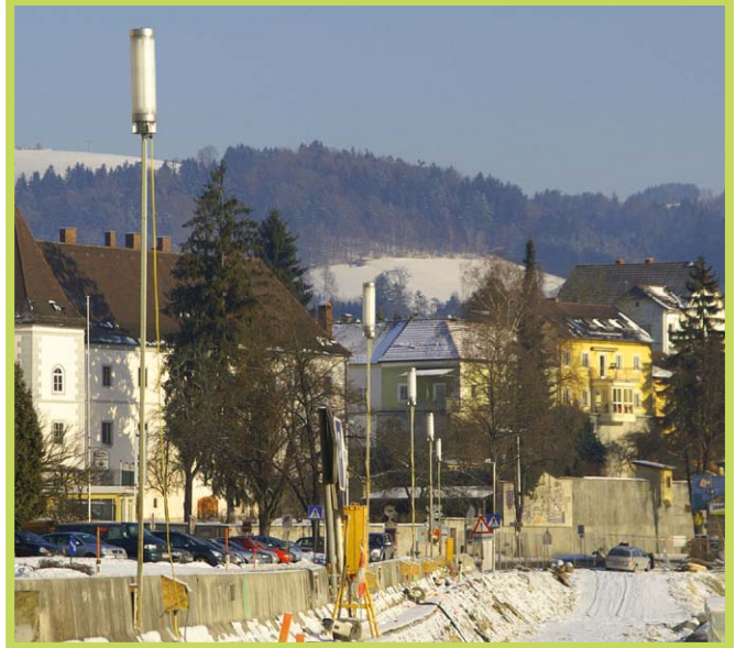
ApolloLED - Lighting on construction sites
