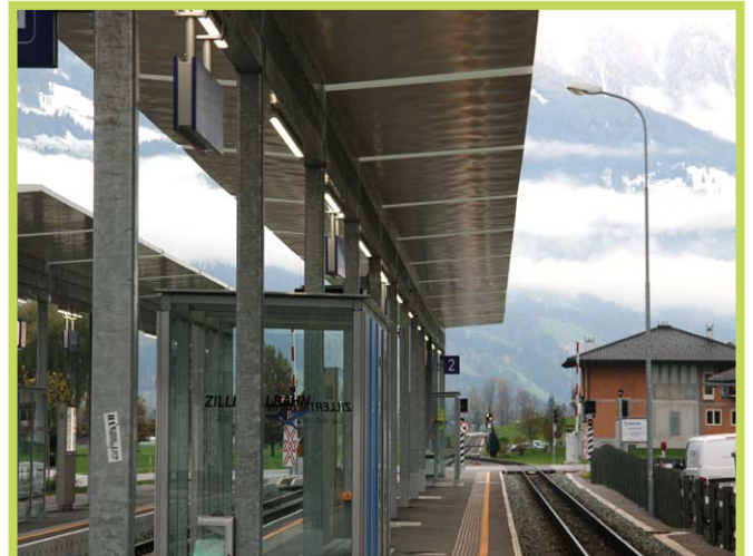
Industry Track LED - Platform / bus stop lighting
