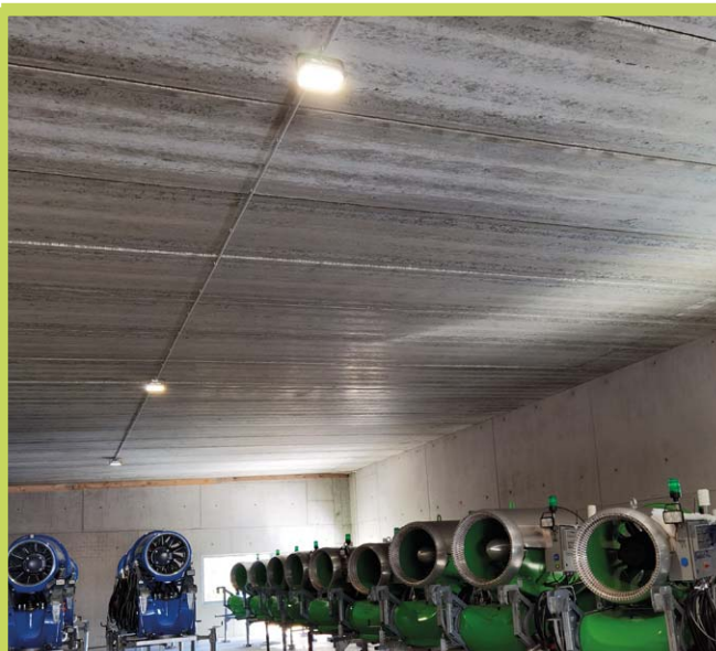
AlphaLUXX - Lighting in the power plant
