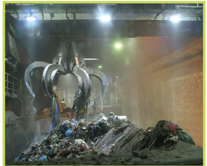
PLAZA - Lighting in waste incineration plant
