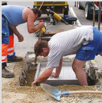
Filling of unit used, and producing a concrete sleeve over all of the stainless steel construction (see technical drawing).
