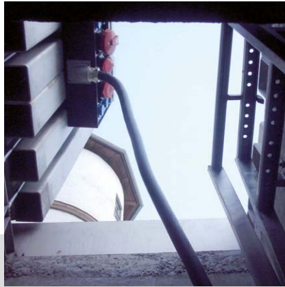
Junkers-Schlössle Götzis: Under-ground distributor PIAZZA 1000 for power supply as well as a manhole.
