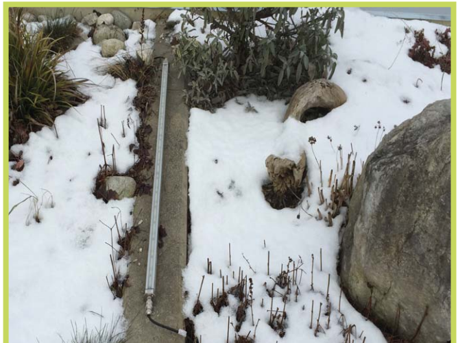
AmbitLED Power - Accent lighting in a plant bed
