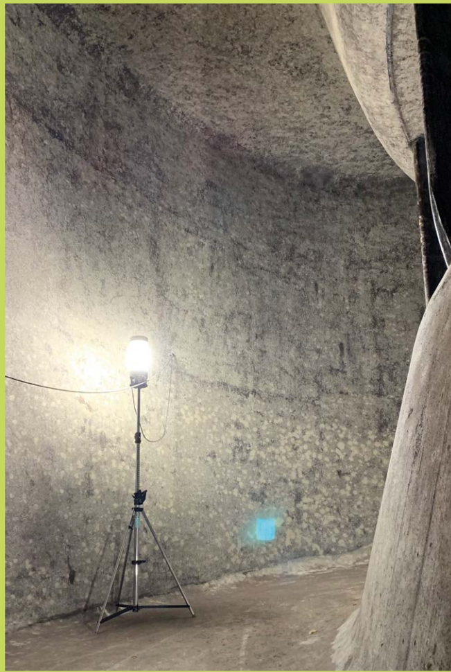
ApolloLED ECO - Lighting during revision work in a power plant
