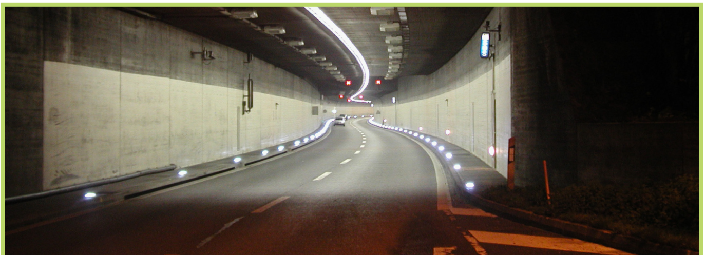
LED guidance systems in the FHS St. Gallen parking garage
