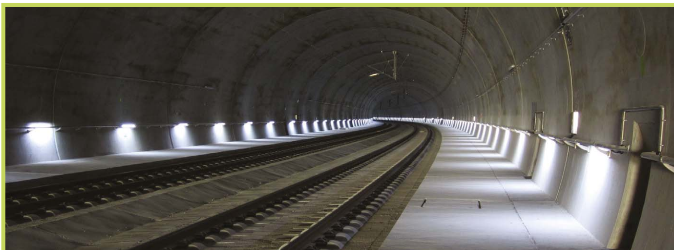
AmbitLED- Lighting the railway tunnel
