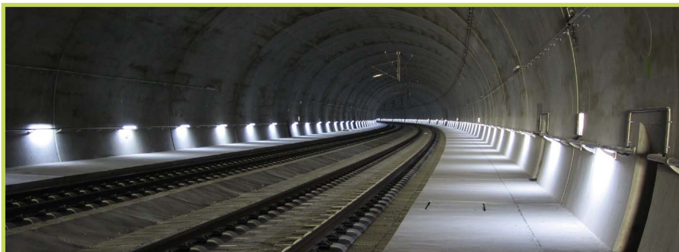
AmbitLED- Lighting the railway tunnel
